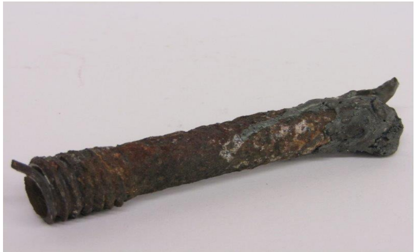
1 of 586 steel stays showing corrosion and the scars of burning out
