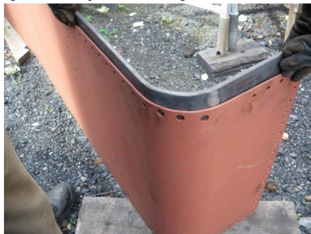
Checking the radius of the butt strip linking upper and lower rear sheets.
